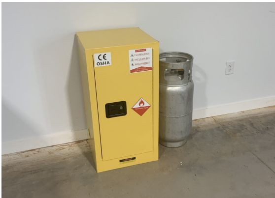
Propane cylinder stored unsecured immediately adjacent to flammable storage cabinet — 29 CFR 1910.101(b)
